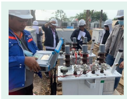
Aux Transformer 5 kVA
