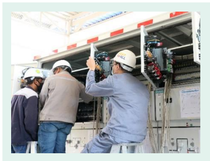
Main Equipment (SWGR)
